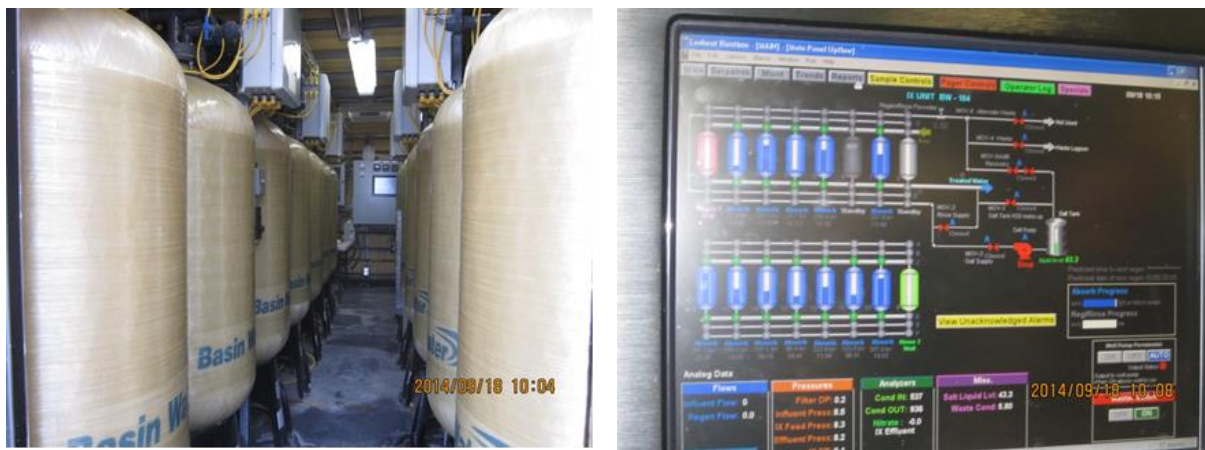
Figure 4-4b Ion Exchange Treatment Equipment (multiple exchange vessels)
